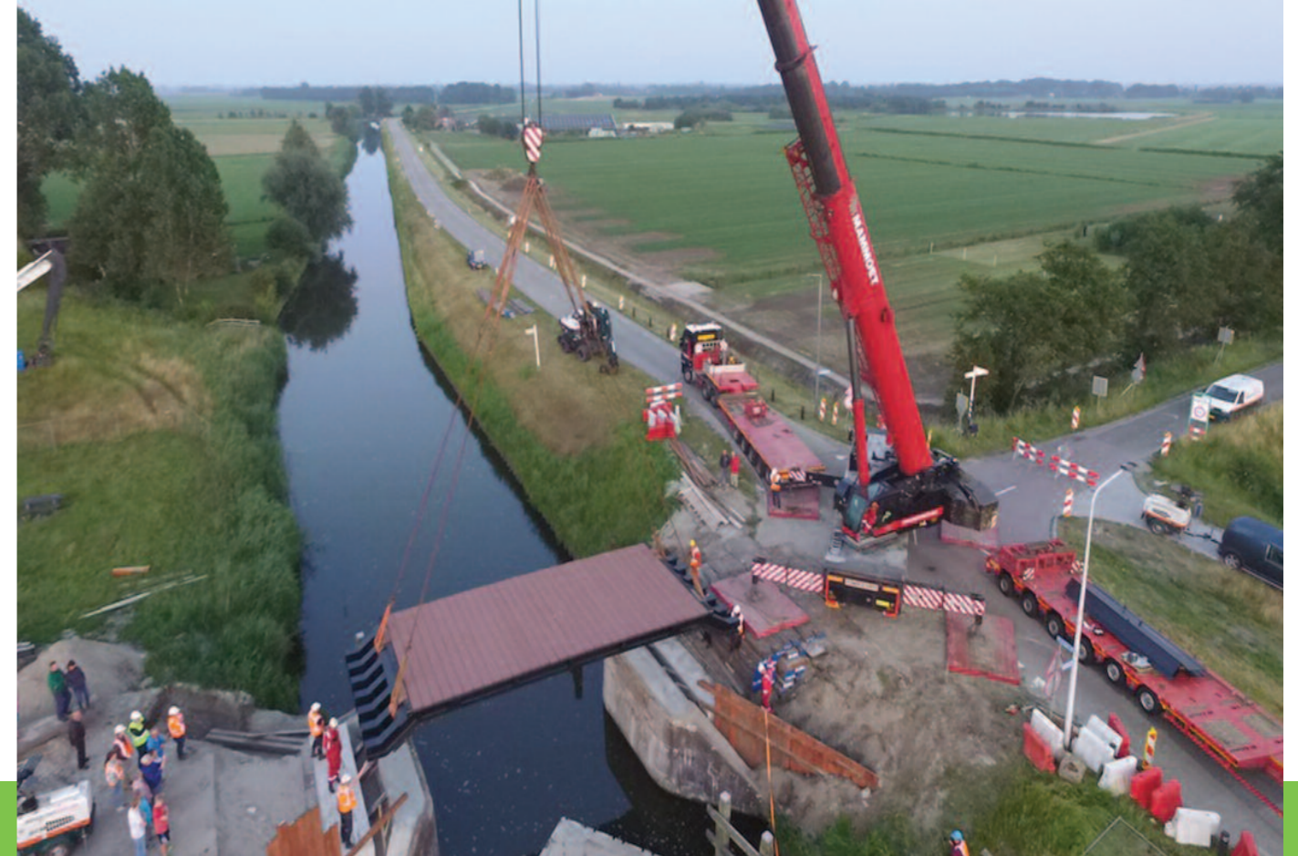
Demacq Recycling International is proud to be a part of this new project – the Dinzerbridgein Dokkum (Friesland, The Netherlands). In the beginning of 2018, our collaboration with Composite Structures has started. The result was a well-designed bridge with a recycled core. The material originated from used train parts made from thermoset composite.
